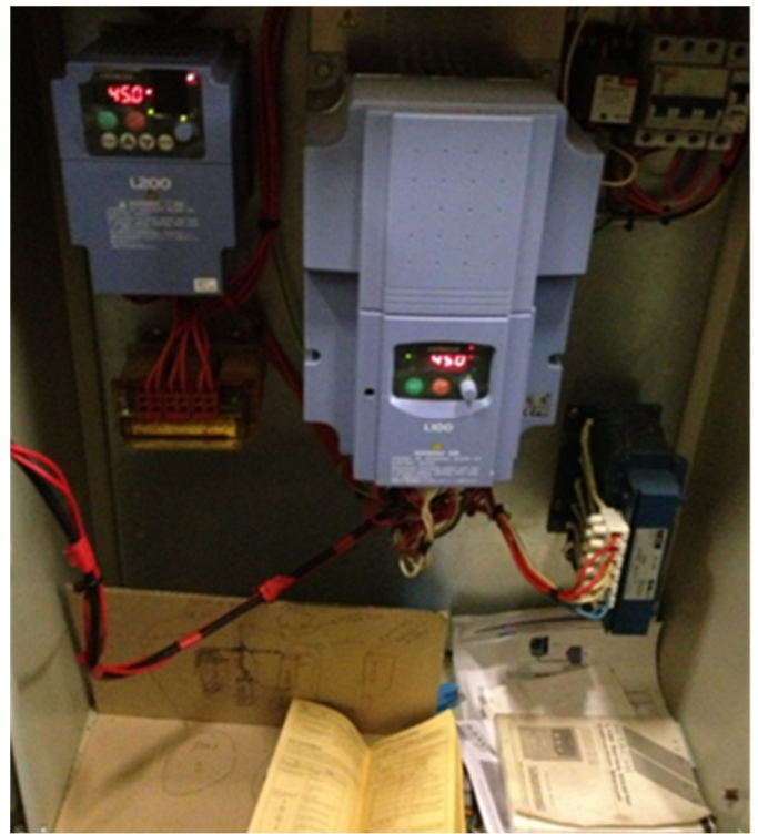
Retrofitting variable speed drives to evaporative fan motors can save an average of $6,000/yr.
